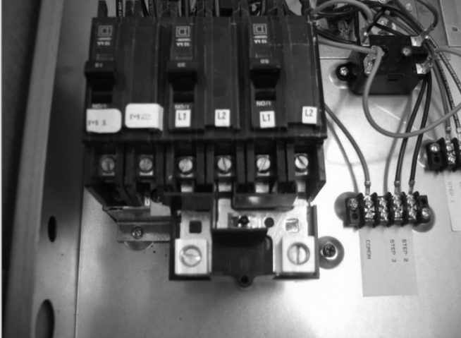
FIGURE 8: JUMPER BAR SHOWN INSTALLED ON CIRCUIT BREAKERS.
